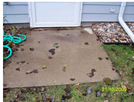
12.) Slab sloped towards home.
