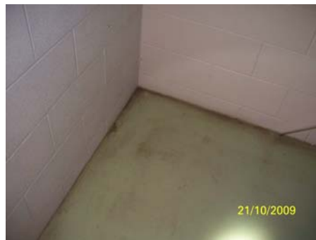
23.) Evidence of past moisture in basement.
